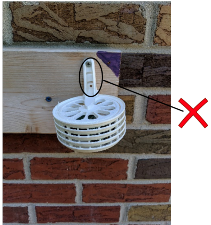
Fig. 8. Incorrect sensor mounting.
